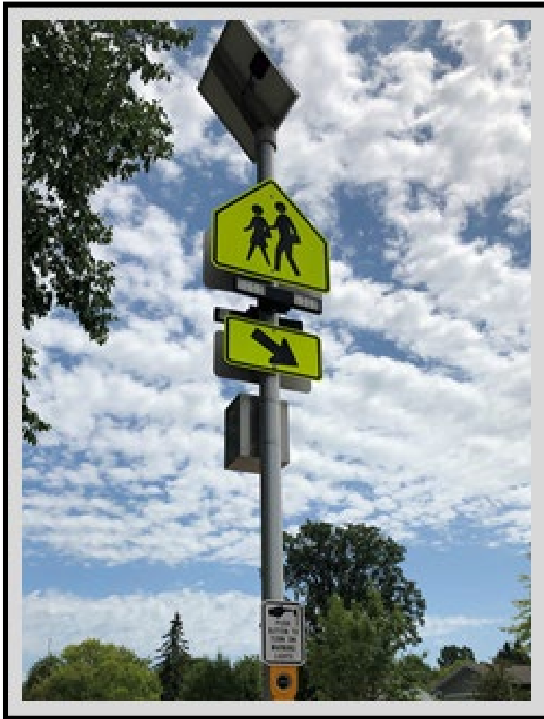
Figure 1. Solar powered RRFB at a school crossing
