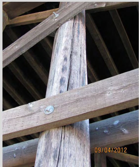
Condition State 3 Surface check extending more than 50% through the pile diameter
