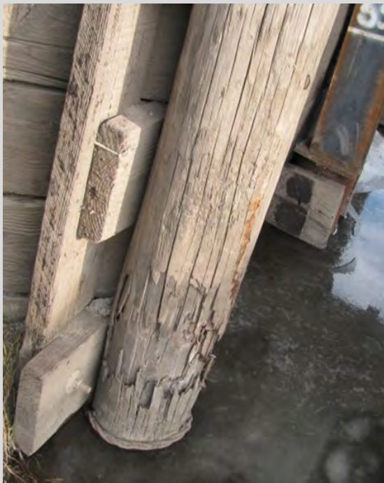
Condition State 4 Shell damage (1" deep) on a timber abutment pile (approximately 30% section loss)
