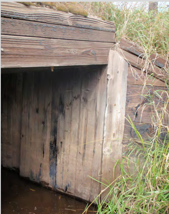
Condition State 3 Wall section misaligned on a timber box culvert
