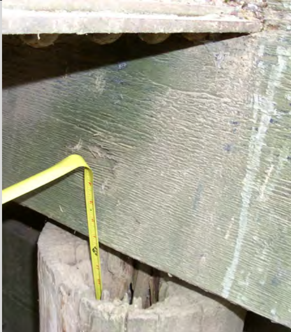
Condition State 4 Severe internal decay (more than 20% section loss) on a timber abutment pile
