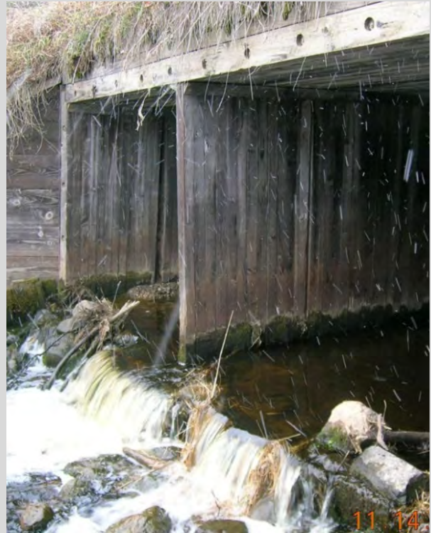
Condition State 2 Evidence of decay along the waterline of a timber box culvert
