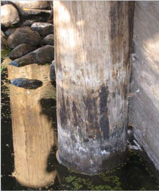
Condition State 2 Timber piling with decay at waterline (less than 10% section loss)
