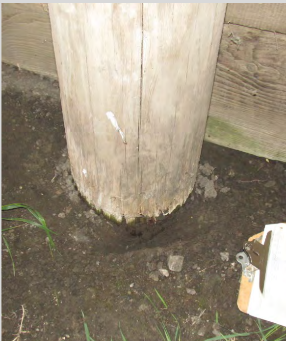
Condition State 3 Shell damage (1/2" deep) on a timber piling (approximately 15% section loss)
