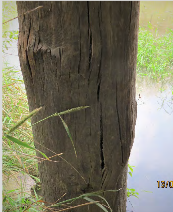
Condition State 4 Timber pier pile is bulging due to crushing (failure may be imminent)
