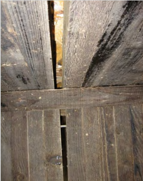
Condition State 2 Separation between timber members on a timber box culvert (no backfill infiltration)
