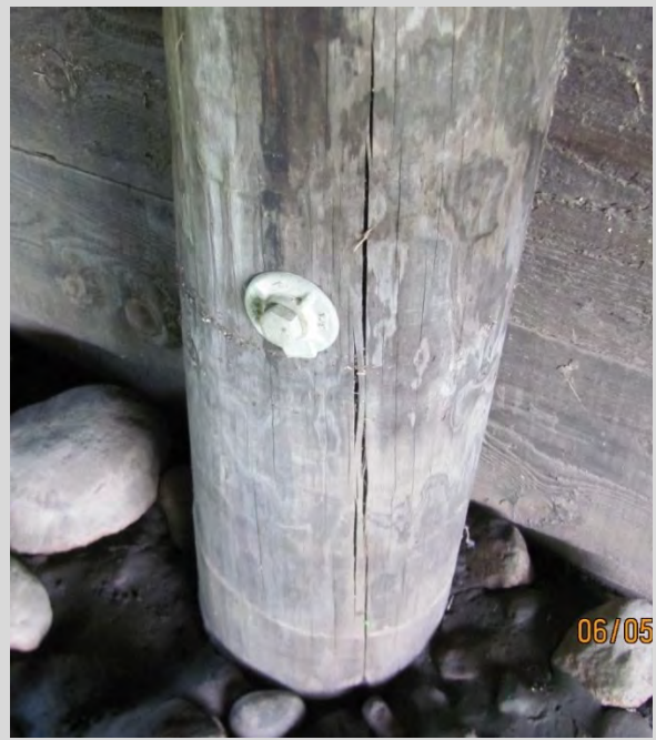
Condition State 2 Surface check extending less than 50% through the pile diameter
