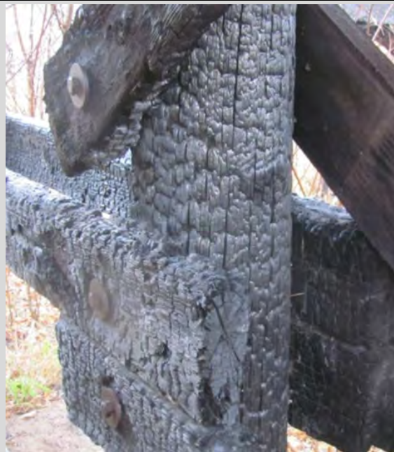
Condition State 4 Fire damage on a timber pile (severe charring approximately 1" deep - 30% section loss)
