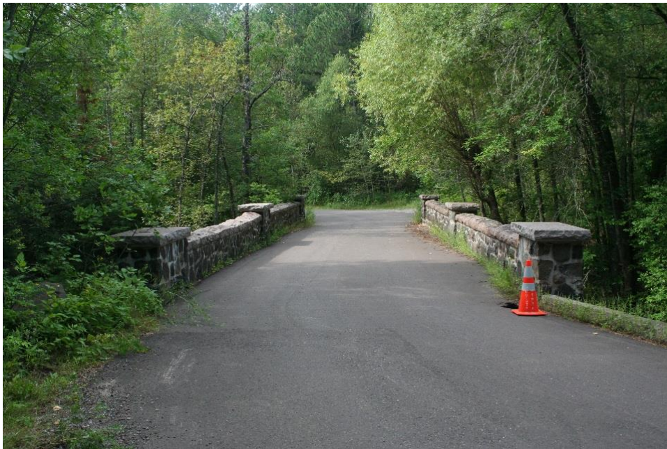
Deck view, top of non-historic concrete retaining wall at far right, view facing southwest
