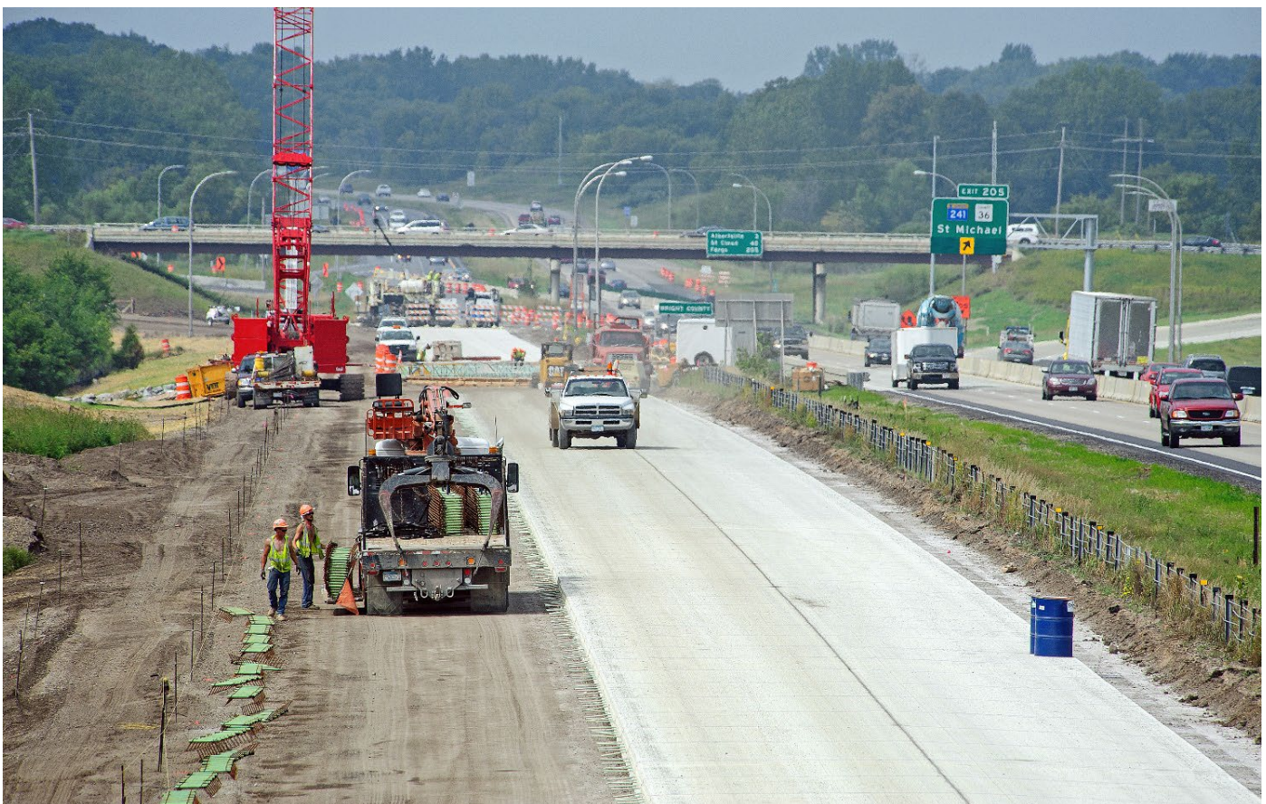
Photo of I-94 Corridors of Commerce project during construction from Rogers to St. Michael
