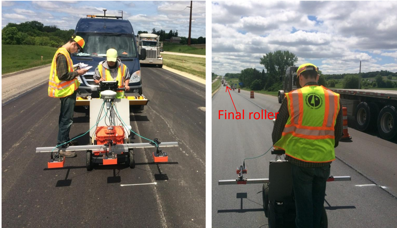
Figure 1. Equipment and Data Collection [A] prior to a 500 ft pass, and [B] during data collection moving behind the final roller compactor.
