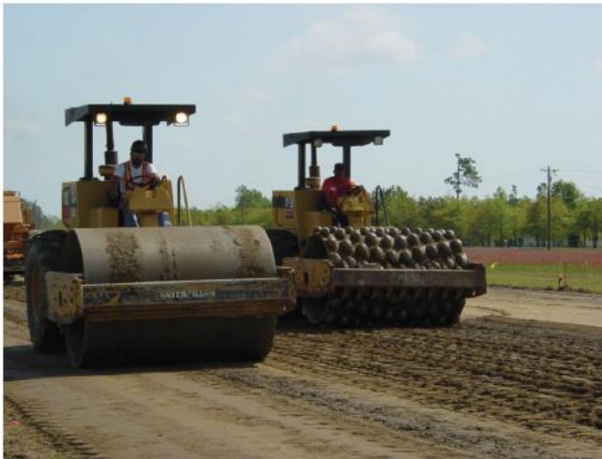
Figure 6. Final compaction of FDR with tamping roller and smooth wheeled vibrating roller [[4]]
